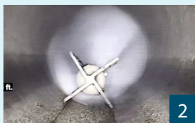
(2) ... cleans the pipes with high pressure water collecting the water and debris via vacuum truck.
