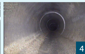
(4) ...takes video for the pipe's length, examining conditions, such as fractures or breaks.
