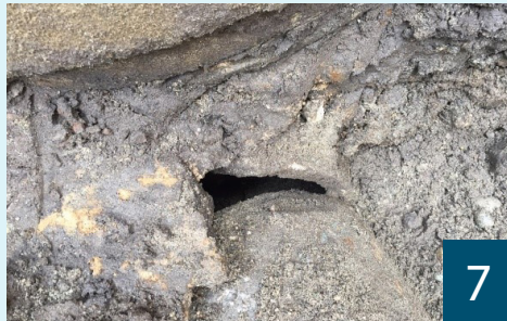
(7) The actual break is located and dug up by Port maintenance crews.
