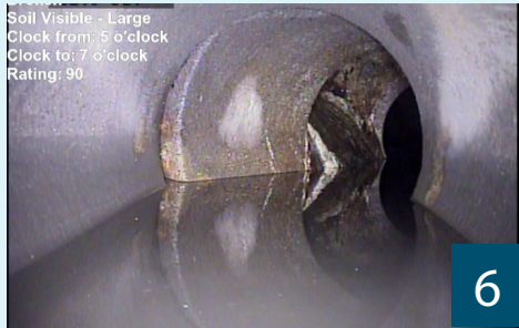
(6) A major break is identified in the pipe. This receives a high condition score.
